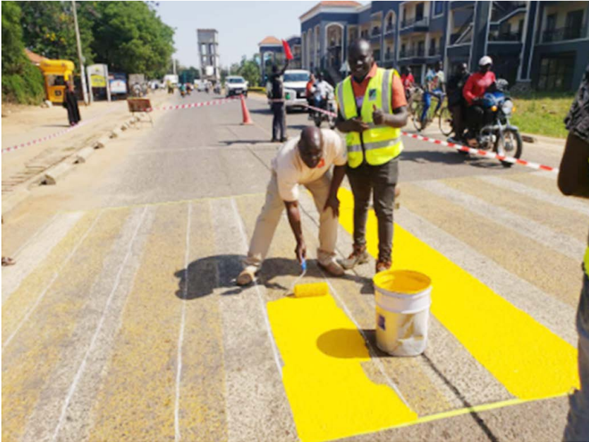
West Nile Regional Members Network Secretary CPA Peter Ijuma participates in painting the pedestrian crossing in Arua City in December 2024.
